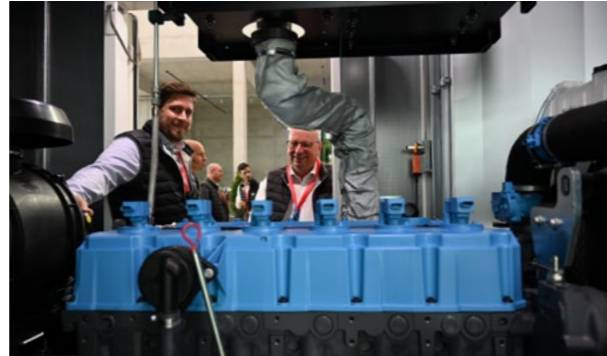
The H2 GenSet produces green electricity.
